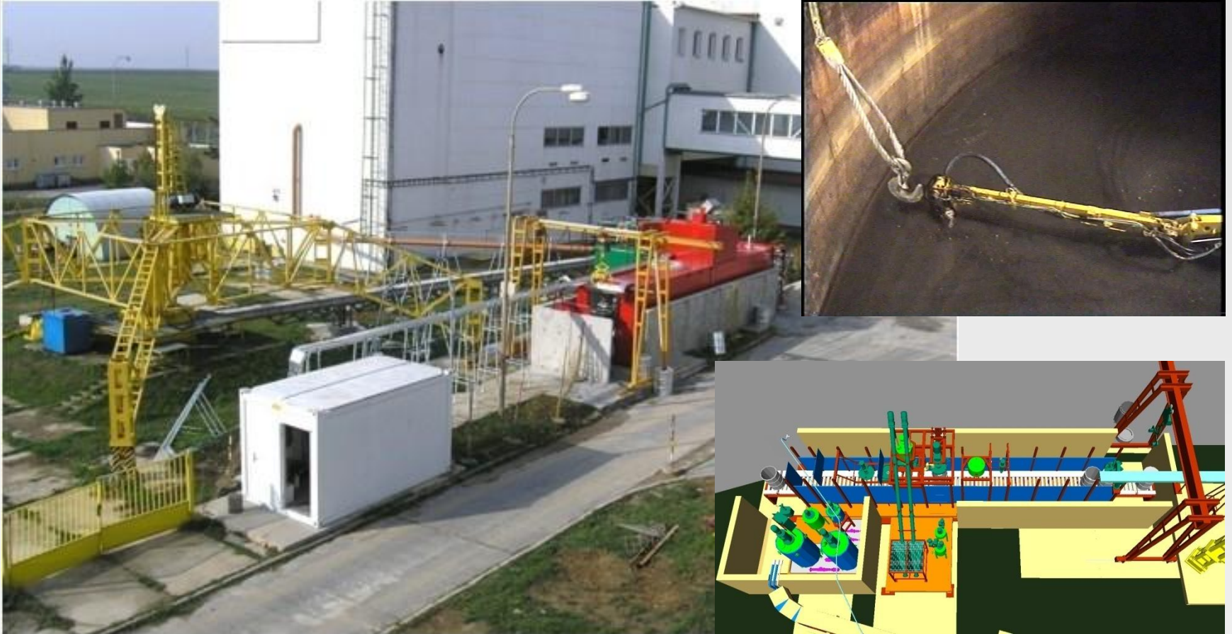
Movable Cementation Facility
